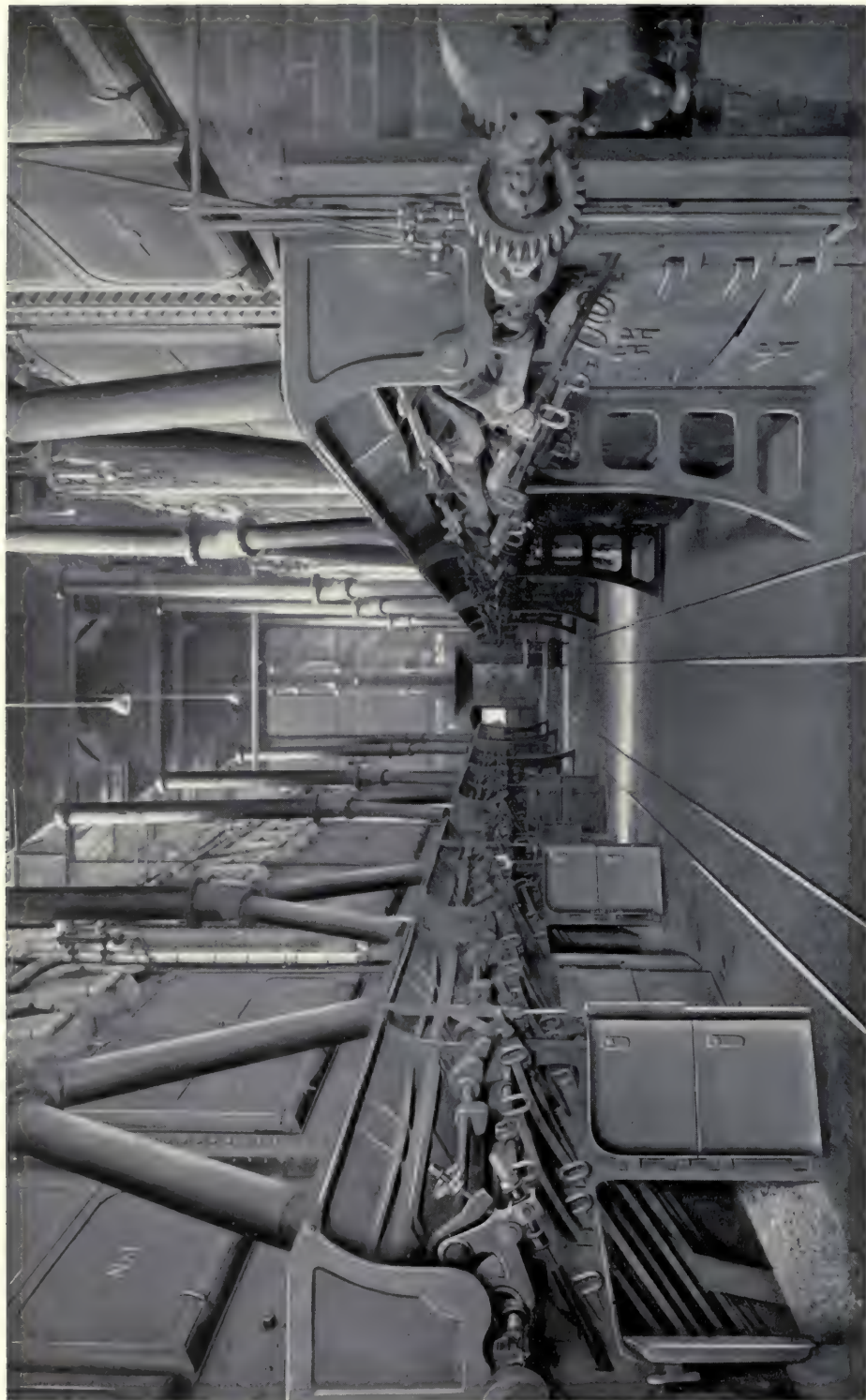
CAPITAL TRACTION CO., WASHINGTON, D. C., OPERATING 7200 HORSE POWER OF BABCOCK & WILCOX BOILERS, EQUIPPED WITH BABCOCK & WILCOX SUPERHEATERS
